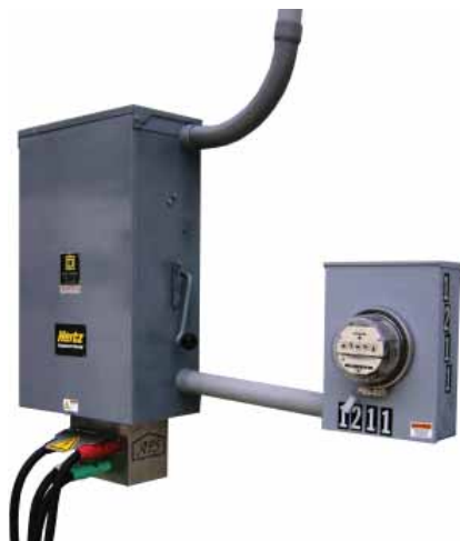
Mounted to Transfer switch
